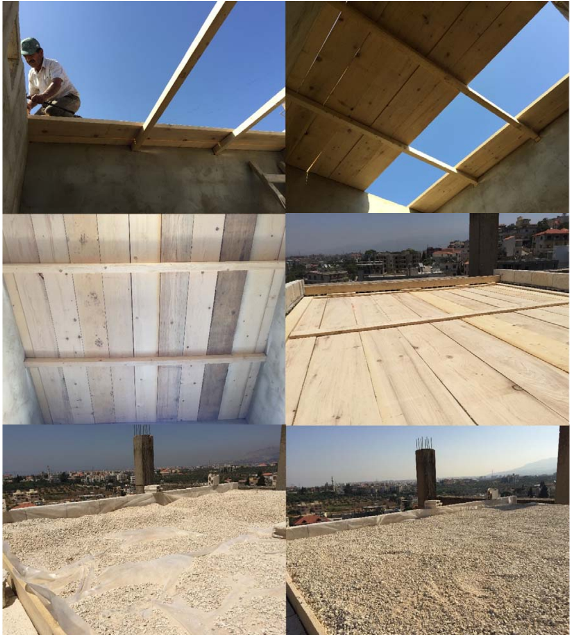
Figure A5.8 Roof progress with the 49mm wood planks above which a thin layer of nylon and 160mm of fine gravel.
