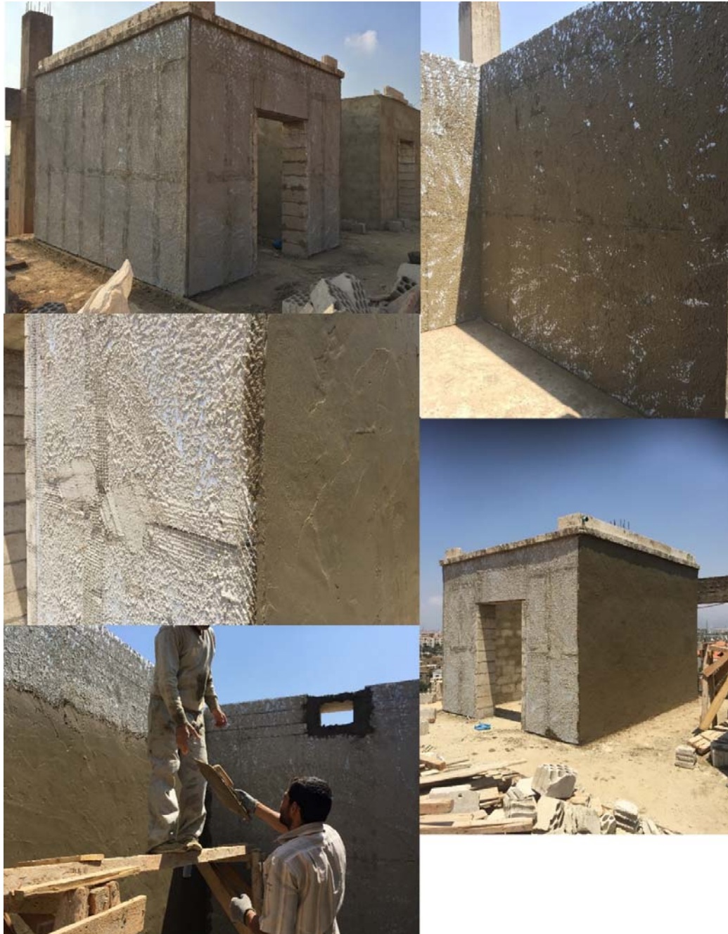
Figure A5.7 Plastering process, showing the first rough surface layer, the splatter dash, followed by the final thicker and smoother later. The angular metal lath is shown as well.
