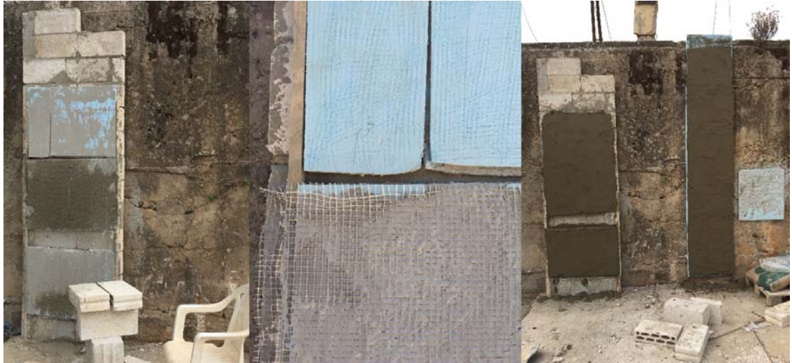
Figure 0.5 Plastering sampling over insulation boards with the surface made rough, and fibre mesh added.
