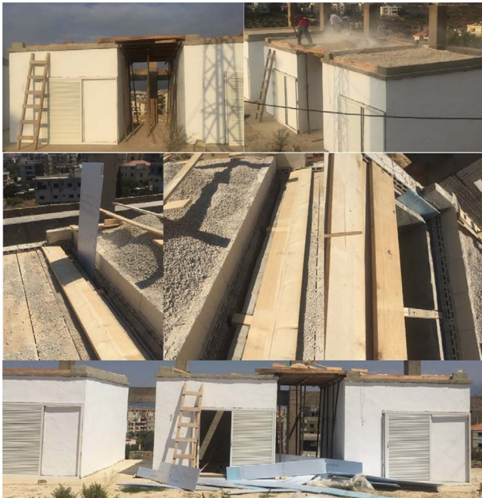
Figure 0.12 Sequence of insulation removal: from the scaffold installation to the gravel transfer, the insulation boards removal, and finally the re-transfer of the gravel and removal of scaffold.
