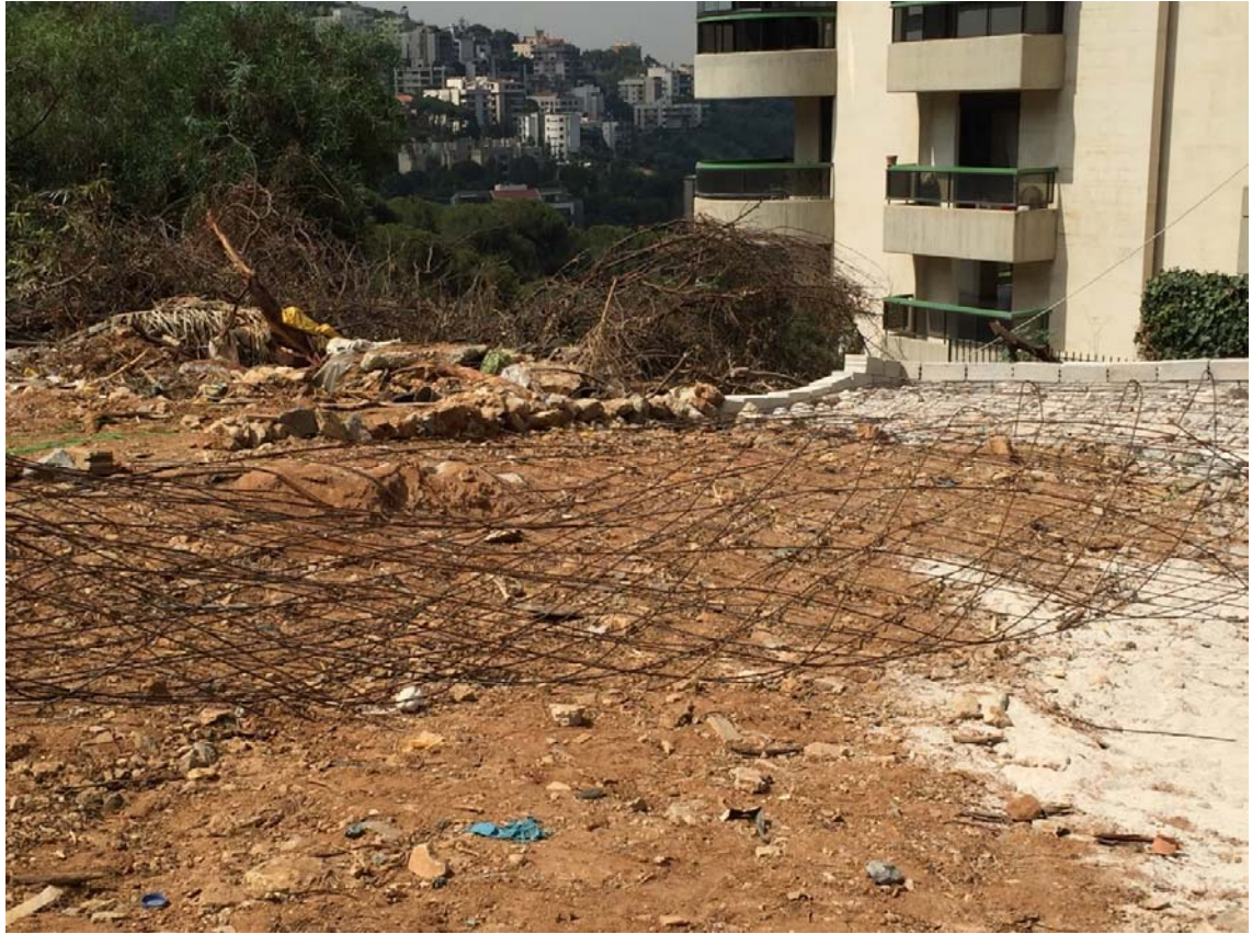
Figure 0.2 The 6mm steel mesh reinforcements torn by the law reinforcement as a statement not to even think of carrying on with the works.
