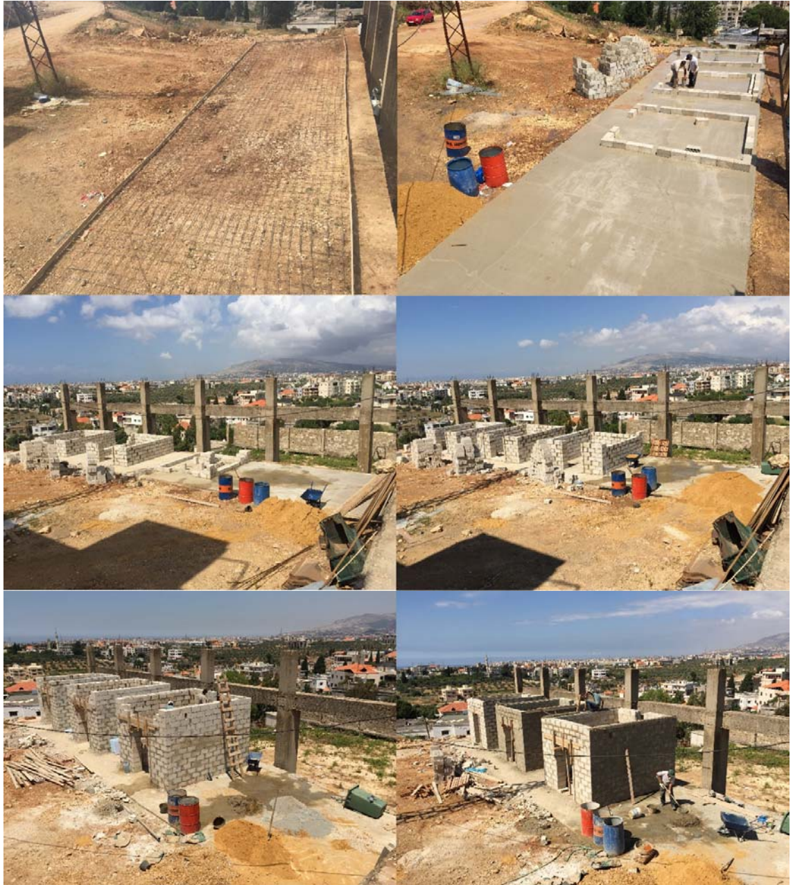
Figure 0.4 Work progress from the clean concrete to the finished 200mm external and 100mm internal concrete masonry walls.
