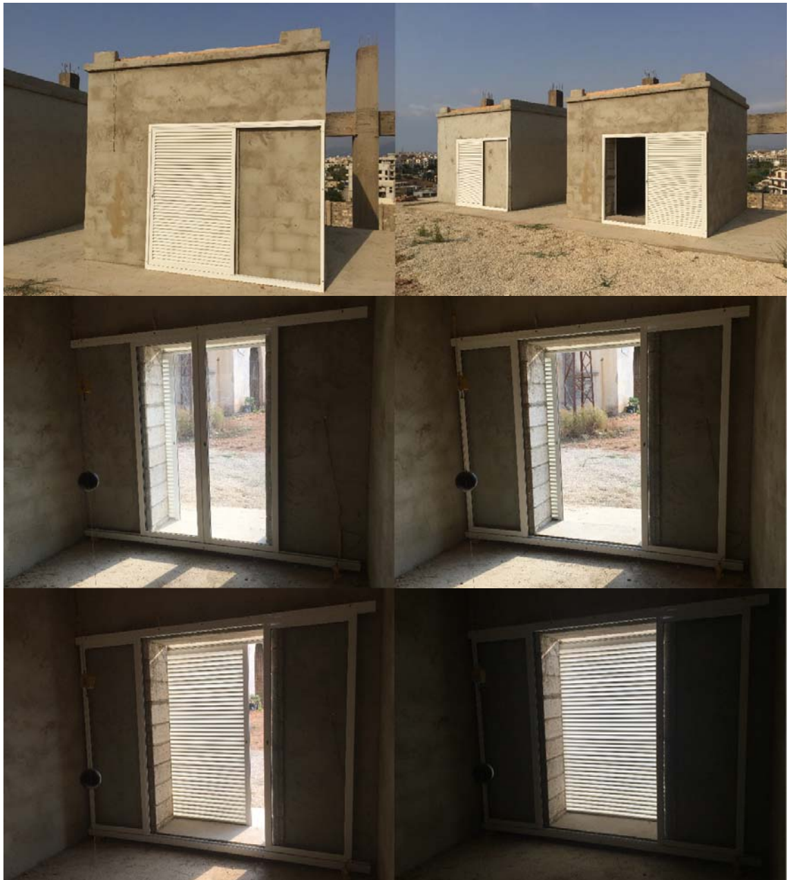
Figure 0.9 The external louvered shutters with their railing frames and the internal two panel single windows sliding on their internal rails.
