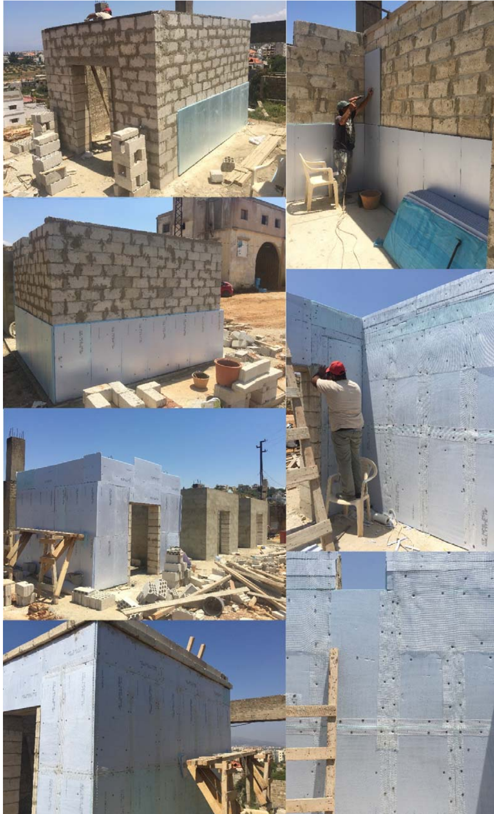
Figure A5.6 Insulation boards fixation, left column externally, right column internally, with screws and wire mesh shown.
